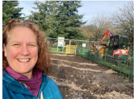
Cllr Abi Mills visiting Greaves Park to see the construction of the new play park she raised funds for.
